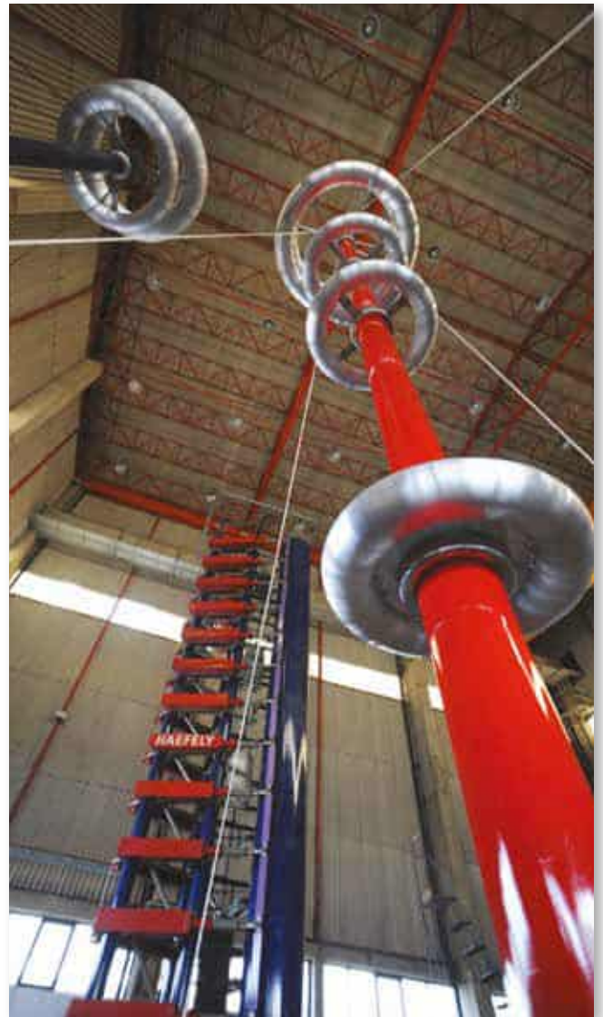
Lightning impulse generator voltage divider.
