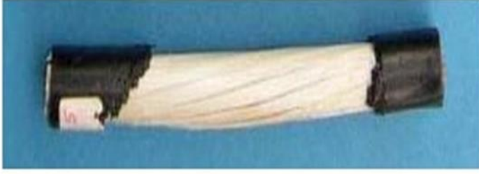
Figure 7: Glass thread protected optical cable exposed to rodent attack
